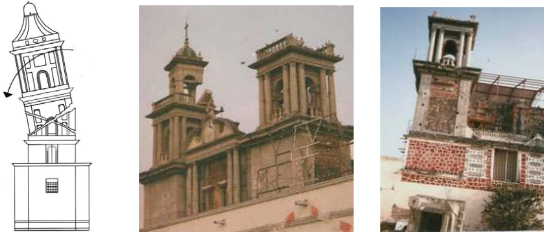
Figure 6 Typical failure mechanisms of bell towers: (Left) [Meli, 1998]; (Right) Effects of the 7.6 magnitude Colima, Mexico earthquake on January 21 st , 2003
