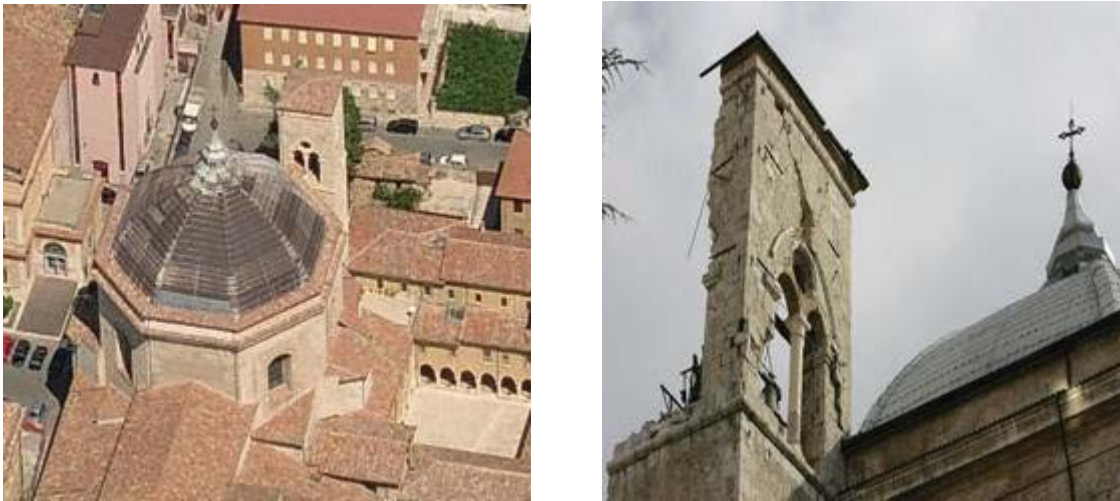
Figure 1 San Bernardino church undamaged and observed damage after the 6.3 magnitude L'Aquila, Italy earthquake on April 6 th , 2009 [Bazrafshan, 2009]
